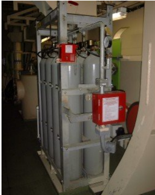
CO2 Scavenge Fire Extinguishing Installation
