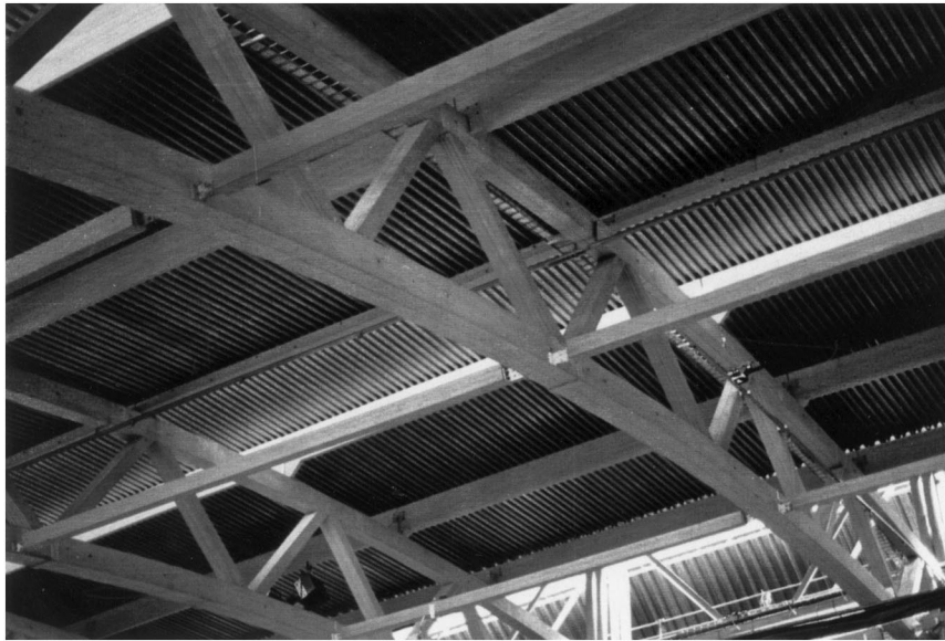
Fig. 12. Timber roof structure of the Olympic hall in Hamar (Norway), span of 250 m.
